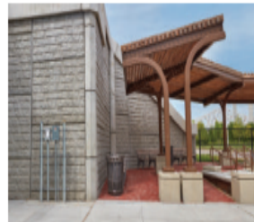
A bike and pedestrian plaza at the Downtown Crossing in Louisville, Ky., features SINE WALL MSE panels.
