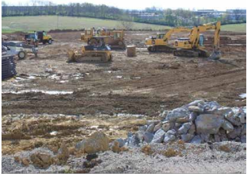
Construction progresses on new State Records Center on Leestown Road in Frankfort.
